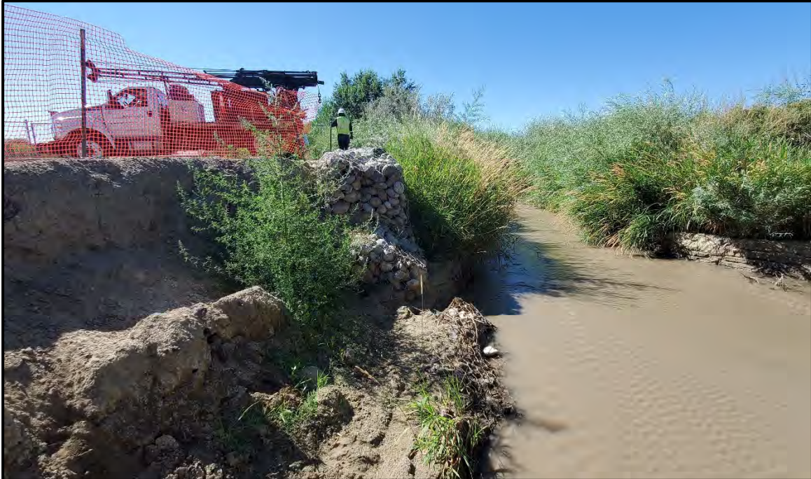
Damaged Gabion Wall near Boring B-3 View Towards the South
