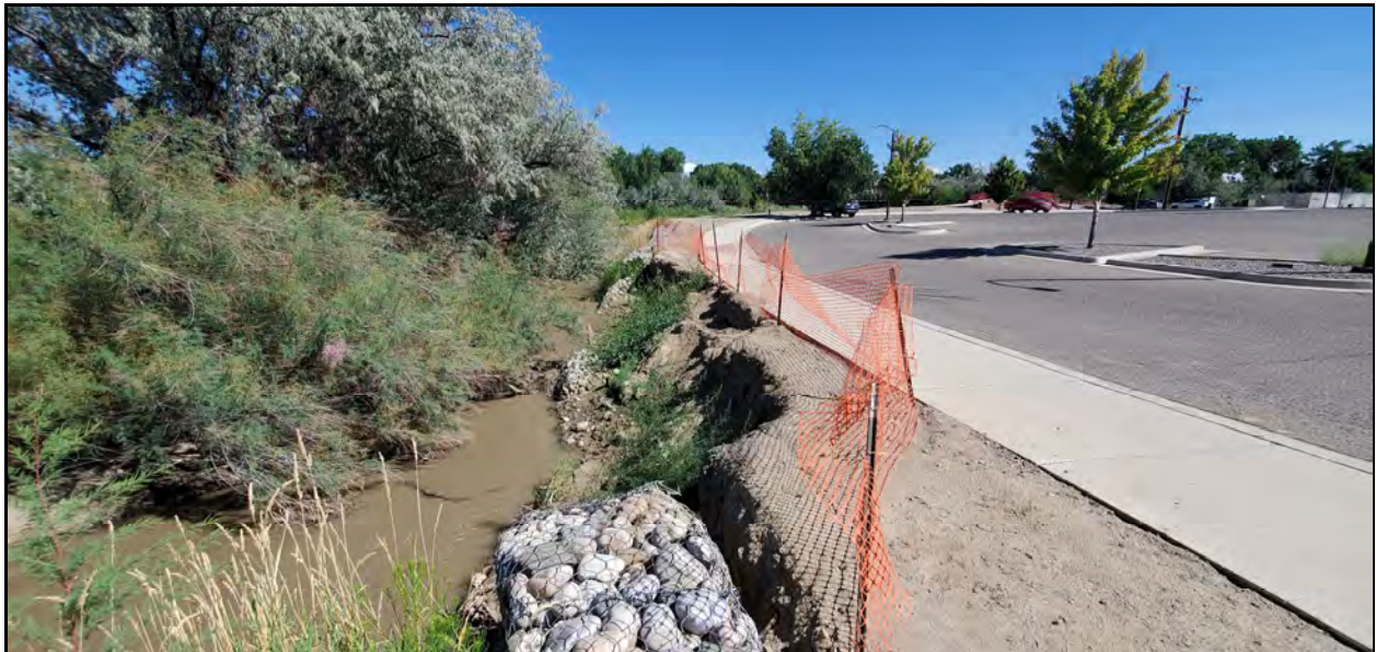
Damaged Gabion Wall near Boring B-3 View Towards the North
