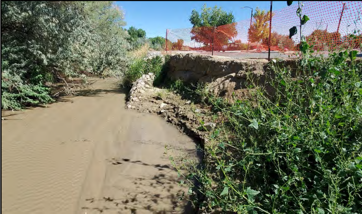
Damaged Gabion Wall near Boring B-3 View Towards the North
