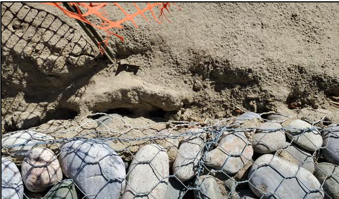
Piping behind Damaged Gabion Wall near Boring B-3 View Towards the East
